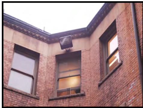
Figure 10: Existing outdoor light.
