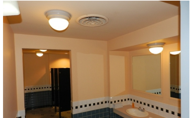
Figure 4: Compact Fluorescent Down Lights and Dome Fixtures
