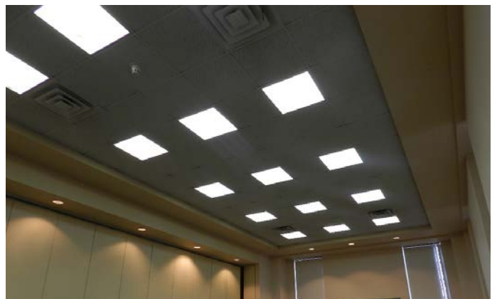
Figure 3: 2'x2' Linear Fluorescent Fixtures with T12 Lamps
