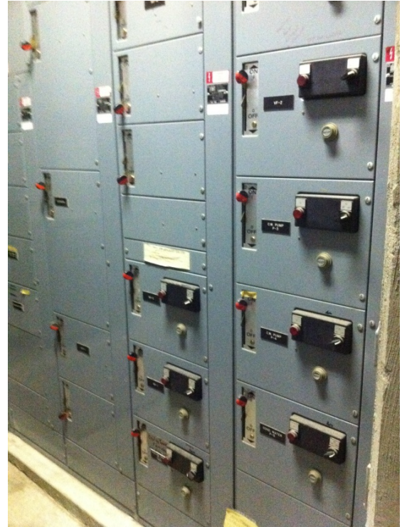
Figure 13: Transfer Switches in Mechanical Room
